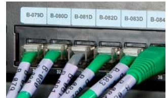
Patch Panel Labels
